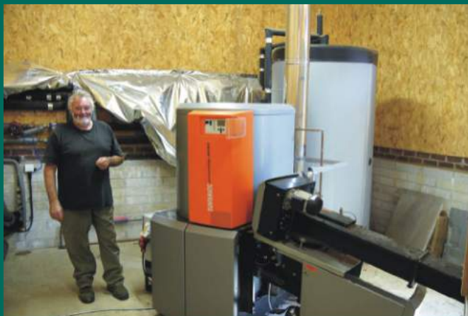
Flint McCulloch by a 35KW woodchip boiler used to heat his new farmhouse using chips from farm hedges and woods. Lewmoor, Hatherleigh, Devon, April 2012.
